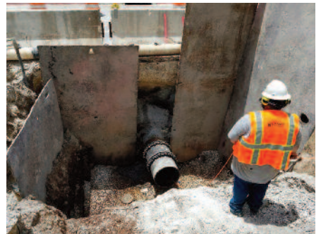
The Insertion Pit was minimal in size and utilized standard MJ assembly
